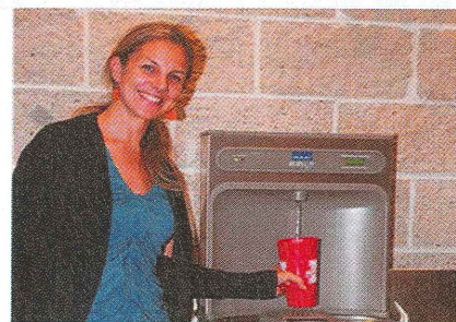
Today, a total of 48 EZH2O Bottle Filling Stations are installed on the Muhlenberg College campus.
